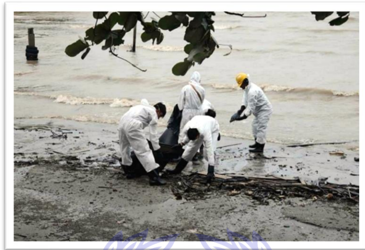
Gambar 1. 4 Cleanup work on the beaches of Sungai Rengit and Teluk Ramunia following the marine fuel spill (MFO) in Pengerang waters, Johor, June 21, 2024
